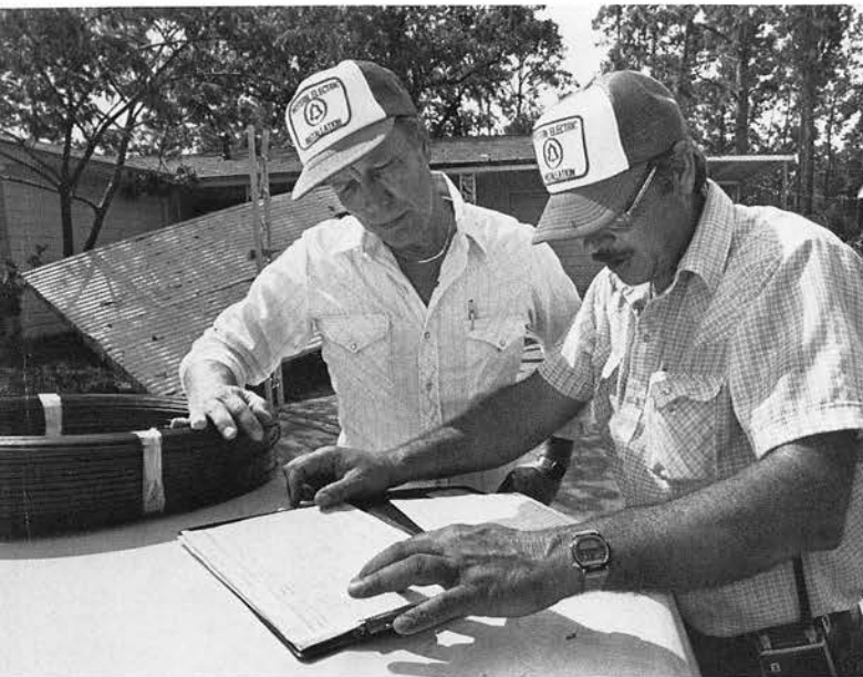
The day after the hurricane, Al Steinke (left) and George Polk, Western Electric installation supervisors, pitched in to help Southwestern Bell repair outside telephone cable.
